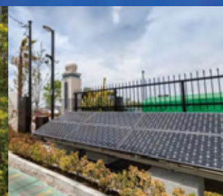
Smart community solar power generation system provides power to residents in the event of an emergency
